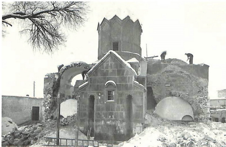
The church of Kathoghike in Erevan : Demolition of the basilica around the small church.
